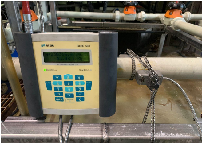
Figure 2: An Ultrasonic Flow Meter
